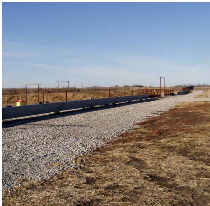
David installed an access road and feed bunks to his cattle pens. The pens will allow David to scrape the pens regularly and apply the manure to his crop fields to utilize the nutrients..
